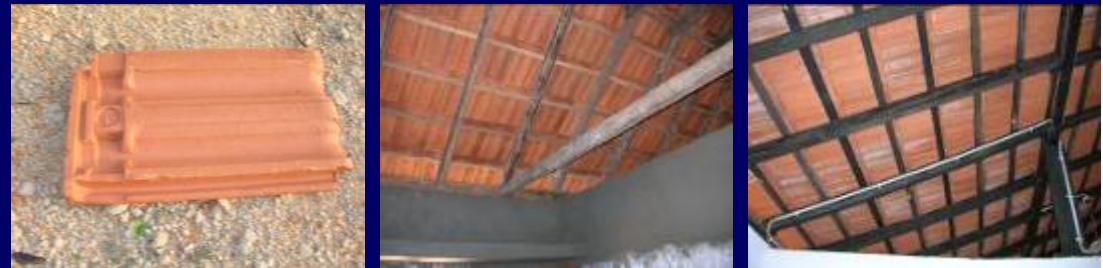
Interlocking tiles not tied to battens or roof frame, but including concrete gable and ridge strengthening.
