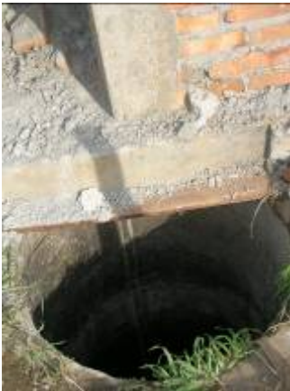
Wall built over Septic Pit
